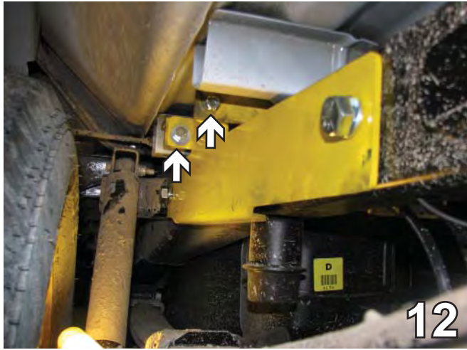
12. Use Loctite on all bolts. Tighten all bolts connecting plate ends to the angle irons (white arrows). Do this on both sides. The driver side is shown.
