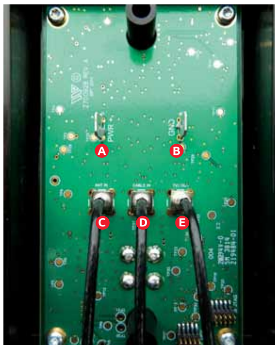
Back of Control Panel
